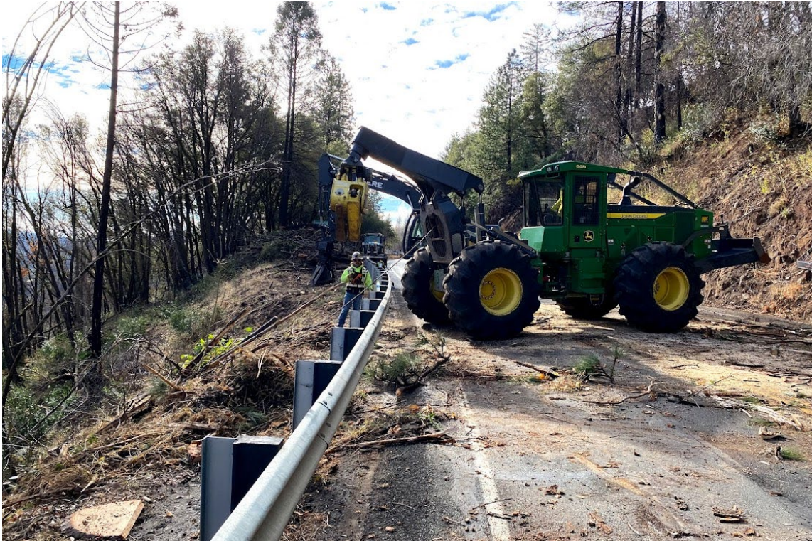
Hazard tree removal on the downhill side of Skyway above aerial tree deconstruction below
