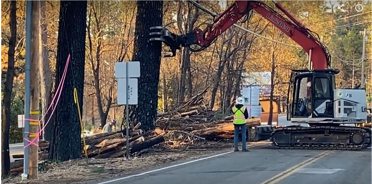
Veteran Faller Chris Blair executing a complex hand fall with mechanical assist – large timber against a communication line.
